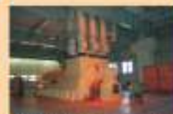
2500MVA Short Circuit Generator
