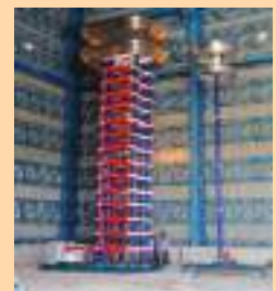
2400kV, 240kJ Impulse Voltage Generator
