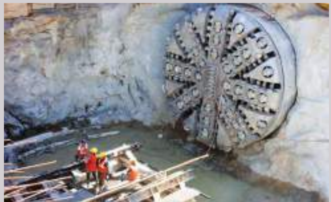
Extensive work on digging tunnels to expand Delhi's metro network is currently under progress. (Photo: PI/Shutterstock).
