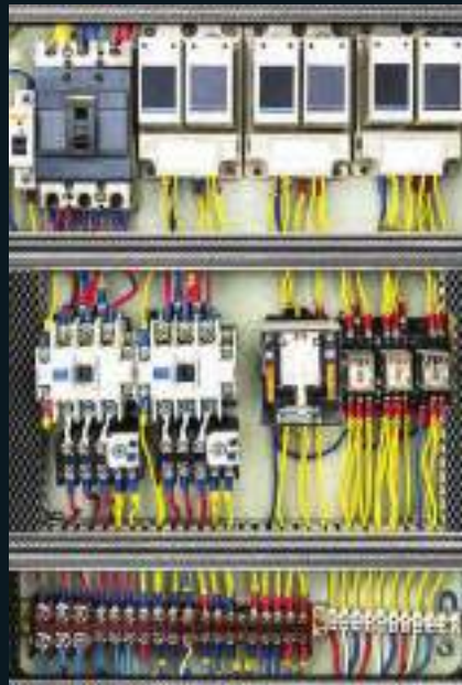
Switchgears are often affected by overheating, which can damage the equipment. (Photo: fotoslaz/Shutterstock)
