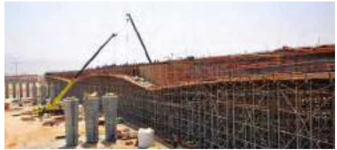
RMD Kwikform was part of a fast-track project to build five bridges in Muscat, Oman. (Photo: RMD Kwikform)
