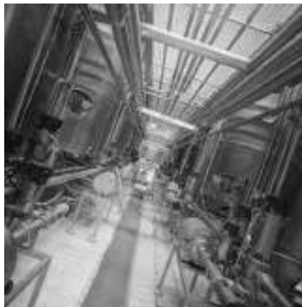
Industrial gases help to keep the wheels of many industries turning. (Photo: Angelo Gilardelli)
