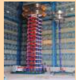
2400kV, 240kJ Impulse Voltage Generator
