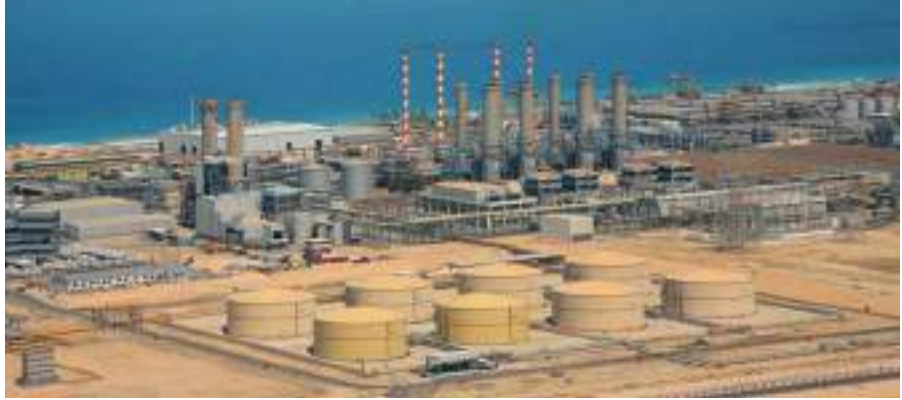
Demand for fresh water from growing population centres throughout the region has resulted in the commissioning of energy-intensive desalination plants. (Photo: Shao Weiwei)
